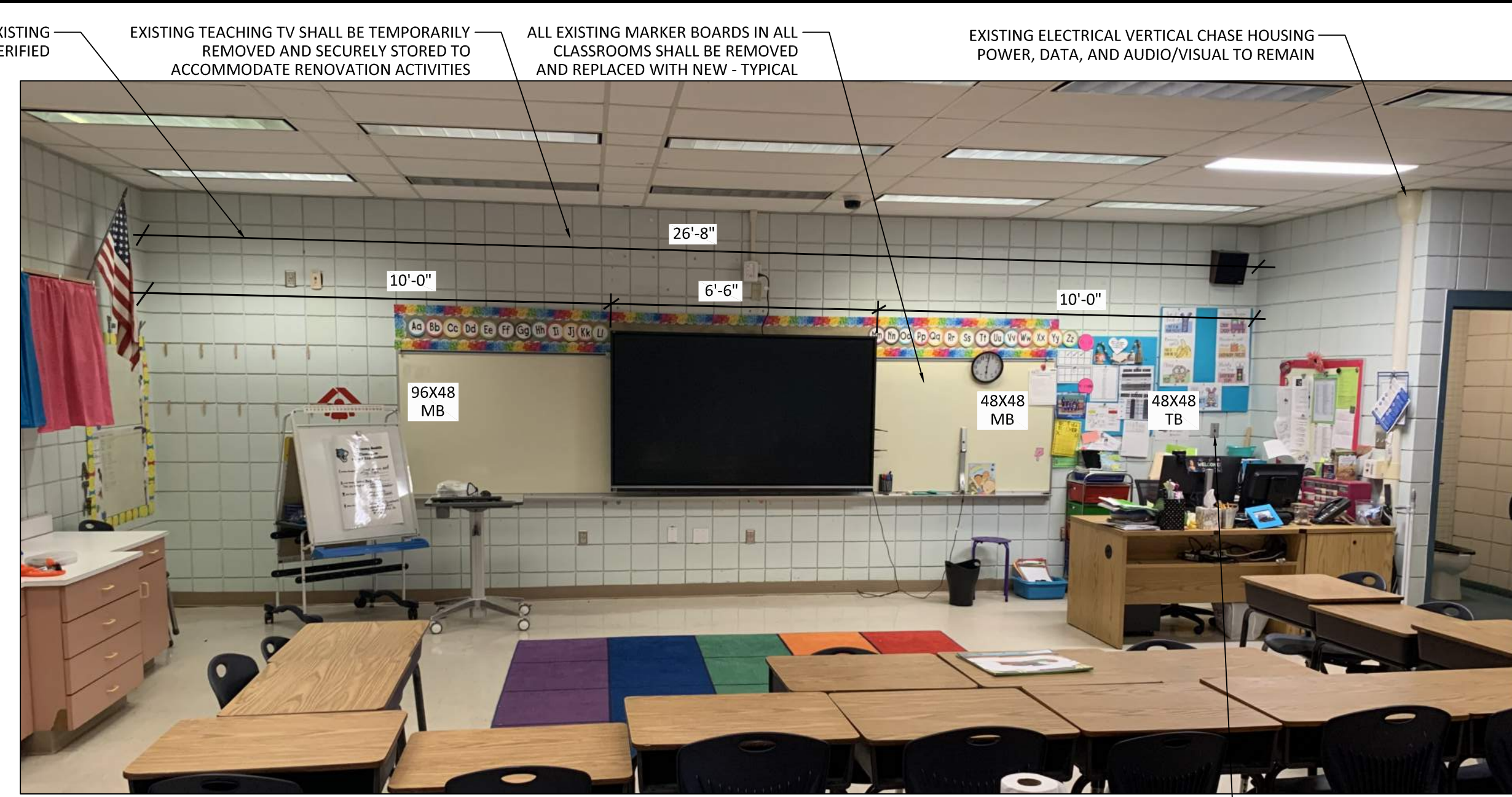
2 CLASSROOM 3-151 TEACHING WALL PHOTO (2-100 SIM.) A301 NOT-TO-SCALE TYPICAL TEACHING WALL CONDITIONS EXCLUDING CLASSROOMS 1-125, 2-114, 2-132, 2-140, 2-148, 3-106, 3-123, 3-143, 3-161
