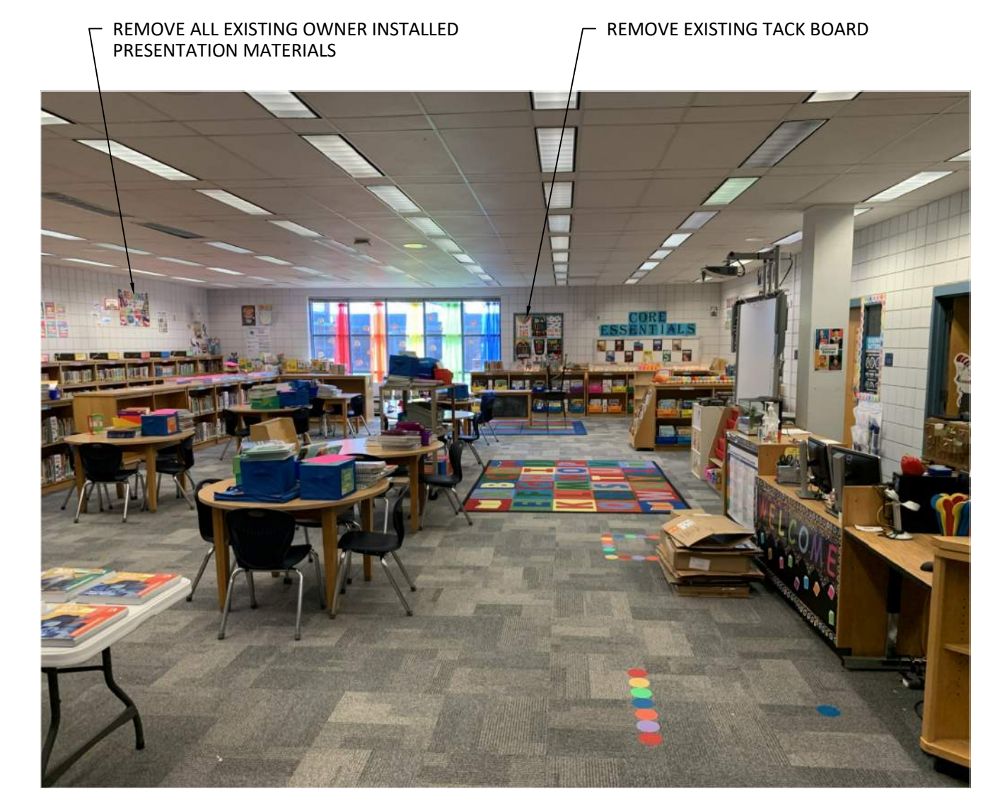
1 MEDIA CENTER - TACKBOARD DEMOLITION AND REMOVAL OF ALL OWNER INSTALLED PRESENTATION MATERIALS 1110 N.T.S.
